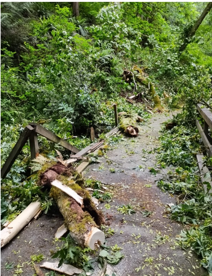
Damage Nature Preserve Bridge #4
