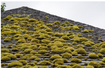
The moss on this roof has taken hold and spread quickly!
